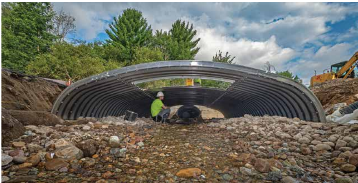
A right-sized culvert replacement in Jay, New York, reconnects habitat and prevents flooding. © John DiGiacomo
