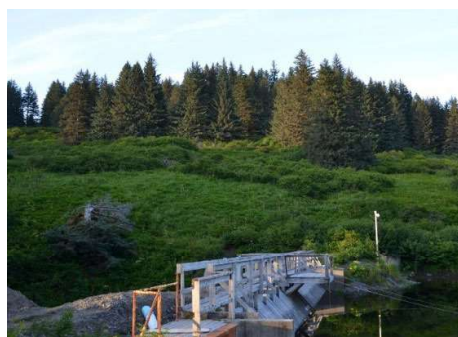
Ouzinkie Dam. Photo Credit: Department of Commerce, Community and Economic Development; Division of Community and Regional Affairs' Community Photo Library.
