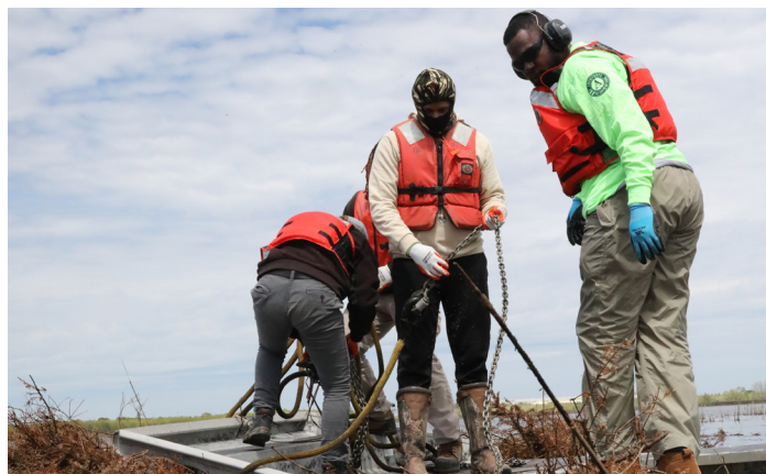
LVI crew members assisting USFWS staff installing Christmas trees to create marsh at Bayou Sauvage. Photo Credit Unknown
