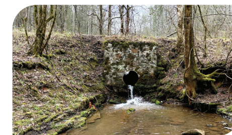
Lowhead Dam at Citico Creek © Lucas Curry/TNC; Undersized Culvert at Citico Creek © Lucas Curry/TNC; Smoky madtom © iNaturalist/Robert Lamb
